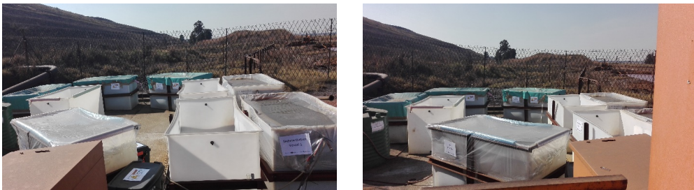
Figure 3 (1 and 2) AMD remediation pilot plant at mine dam site (photographs taken by authors)
