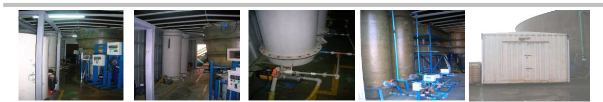
Figure 6. ZEOTREAT technology pilot plant
