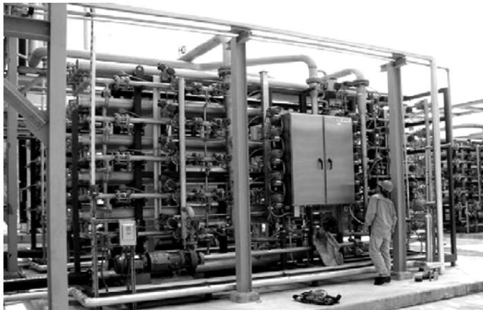
Figure 2 PPPWTS RO membrane skids
