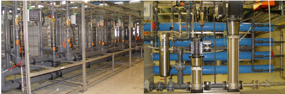
Figure 2 ED (left) and RO (right) in the GEAM plant (Toman 2009).
