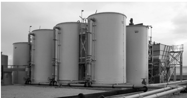
Figure 1. Horden Colliery HDS mine water treatment plant with the reactor tanks left and the lamella clarifiers at the right side (photograph: Andrea Hasche).
