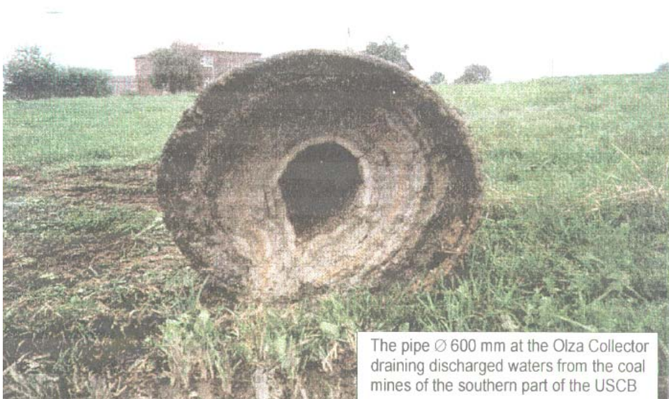
Figure 1 The deposit made in pipe of the Olza Collector
