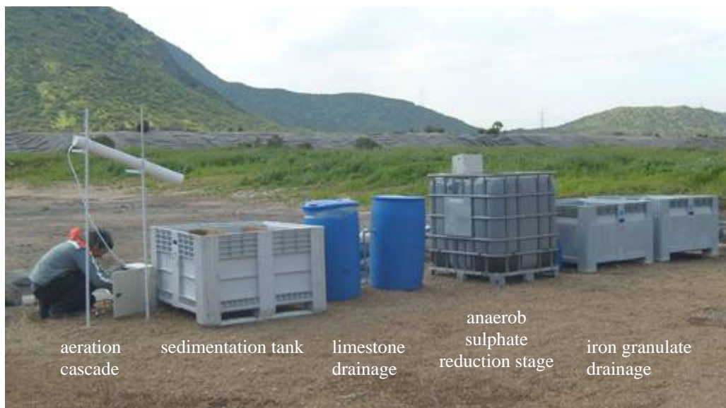
Figure 7. pilot plant for the passive biological treatment of sulphate loaded leachate using a Constructed Wetland at the Lo Aguirre mine
