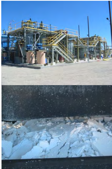
Figure 2 IX treatment option for removing high sulfates and the Gypsum bi-product (BioteQ's Sulf-IX™ process plant)
