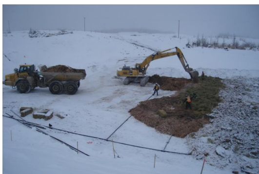
Figure 1 Construction of the field-based BCR showing the perforated feed pipes, organics (brown) and rock (right-hand side) layers.
