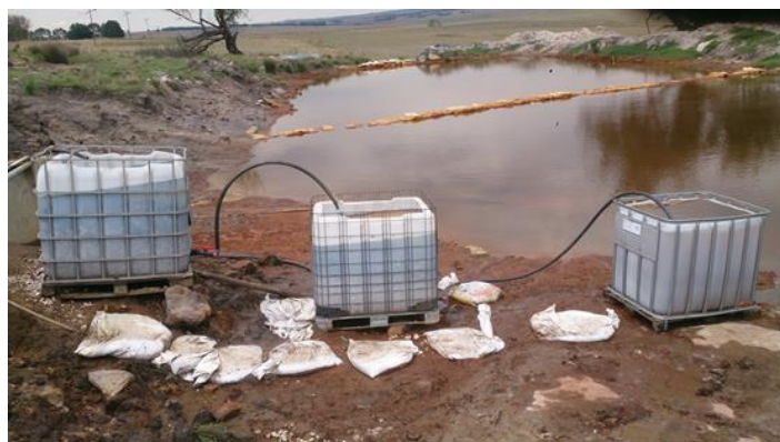
Figure 2 Carolina pilot passive treatment RAPS and oxidation units
