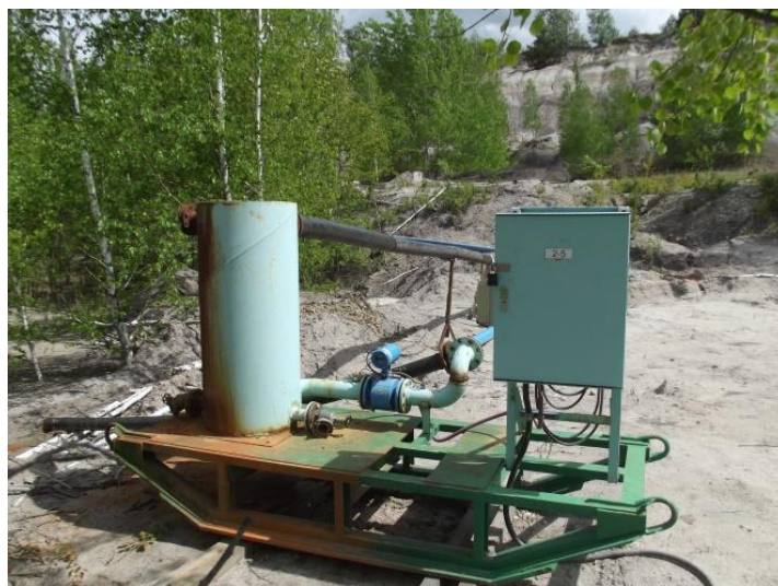
Figure 6 Measuring device of the HDD well.
