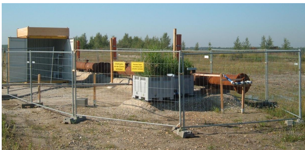
Figure 4 Pilot plant at former lignite mining site
