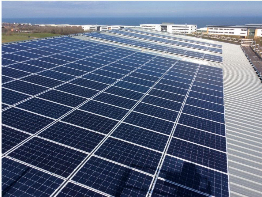
Figure 1 Dawdon active scheme 49.92Kw scheme installed in 2016 consisting of 192 260 W panels.
