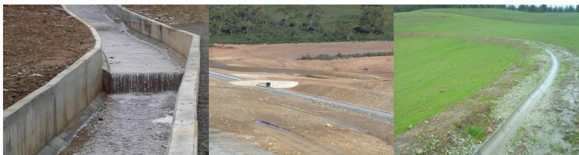
Figure 7 Aljustrel cleanwater diversion channel and Vale d'Abrutiga surface run-off drainage system.
