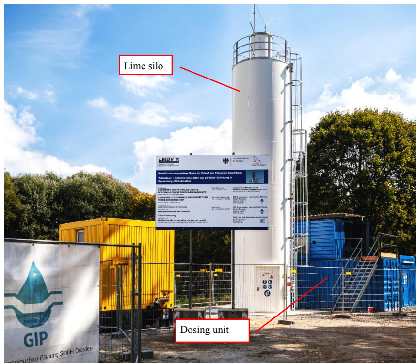
Figure 2 Container-based mobile plant providing tailored lime slurry dosing (Plant Unit 1)
