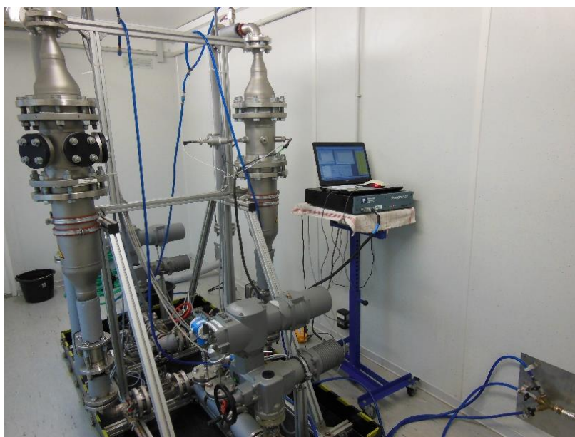
Figure 6 Test bench for in situ precipitation from geothermal brine
