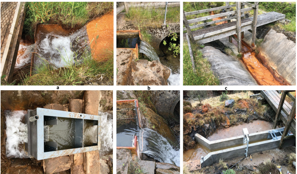
Figure 3 Glyncorrwg MWTS flow monitoring upgrades
