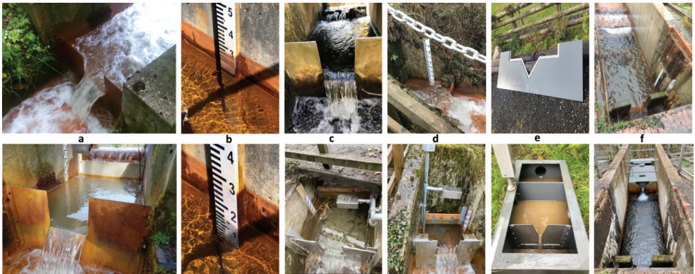
Figure 2 Improvements to primary flow monitoring structures
