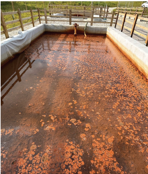
Figure 2 VFR 1 and its aeration rose, showing iron accumulation on the surface of the media layer.
