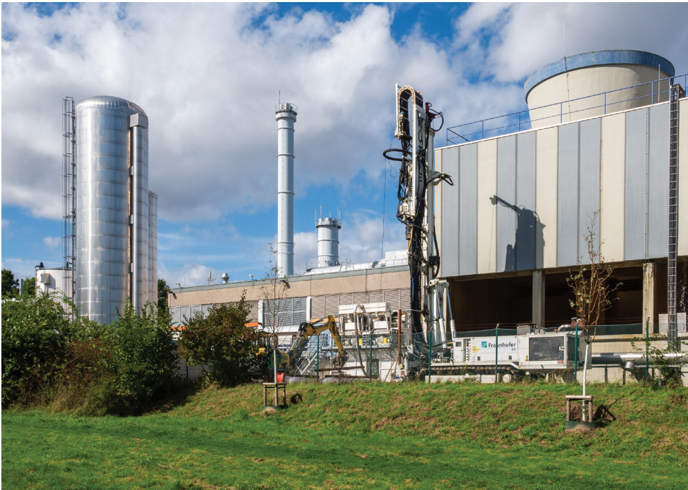
Figure 2 Drilling rig in front of the Technical Centre's cooling tower (on the right).
